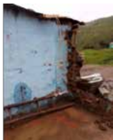
Figure 2: Collapsed house for Khambule family in Ofafa Emashakeni Gquzu area under Ubuhebewe
