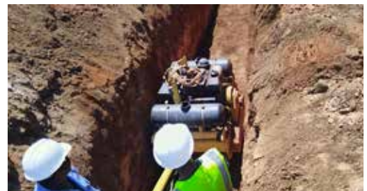
Excavation of the rising main pipeline started, preparing bedding of the pipeline.
