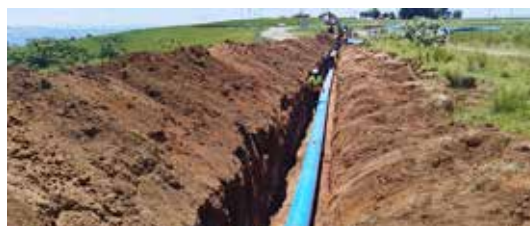
Pipe Laying In Progress, To date the contractor has laid 486m of 355mm diameter pipe, the work was done in three consecutive days.
