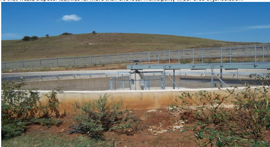
UMzimkhulu Waste Water Works
