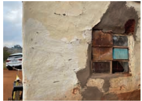
The condition of the house that fourteen people live in.
