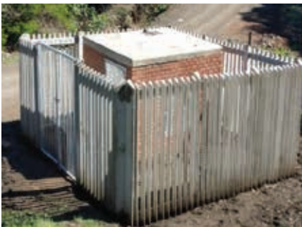
Pump house inside with borehole inside
