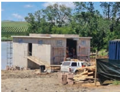
Mbizweni pump house
