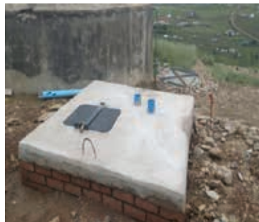
Connection chamber to the existing reservoir
