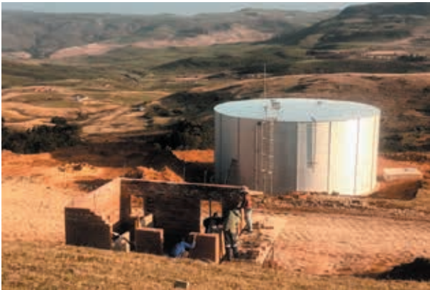
Construction of the Guardhouse at the Package Plant and Reservoir Site in Khukhulela.
