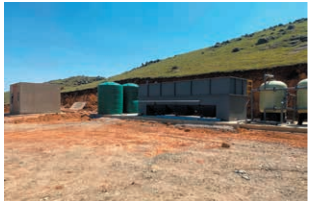
Installed Package plant with the storage tanks
