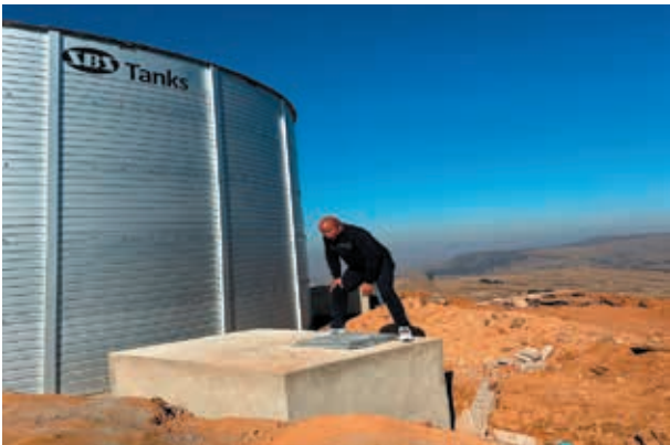
Final Inspections at the 500kl Clear Water Storage Reservoir at the Khukhulela Water Scheme
