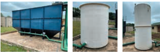
Clarification Zone: Clarifier, Settled Water Tank, and Flocculation Tank – operational.
