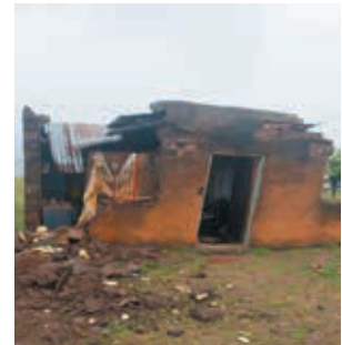
Structural collapse in Ubuhlebezwe, Ward 11 Ndwebu on 17 October 2023 caused by heavy rainfall and strong winds.
