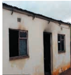
Structural fire in Ubuhlebezwe ward 10, KwaBhidla on 17 October 2023
