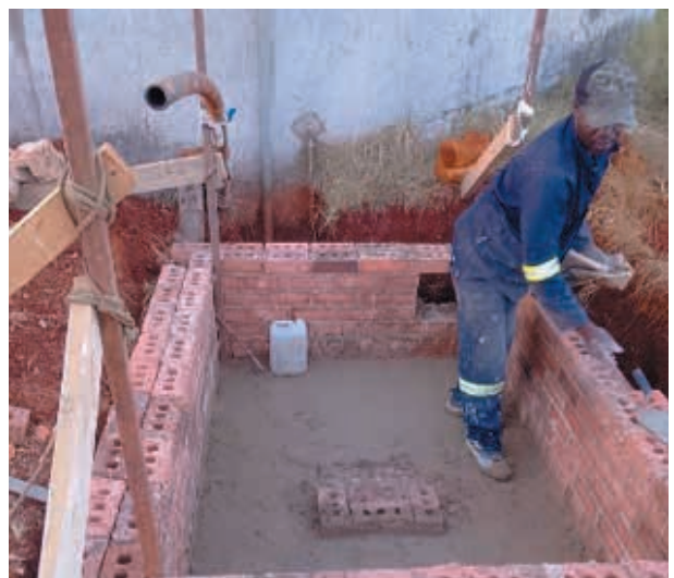
Previous construction of Mahehle command reservoir inlet chamber. Chamber roof slab, specials and pipework to be installed.
