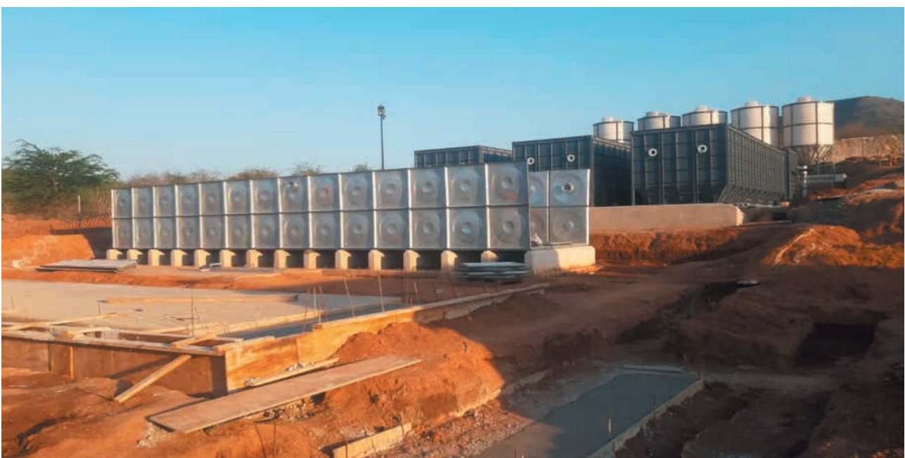
Clarifiers, Coughulation and flocculation tank, Backwashers, Clearwater storage tank, preparation of sand filters platform and chlorine building room
