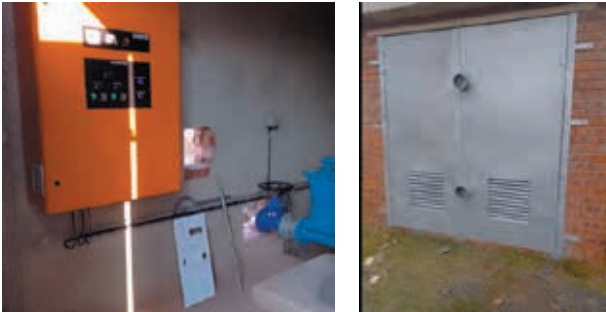
Abstraction PS – completed and operational.
