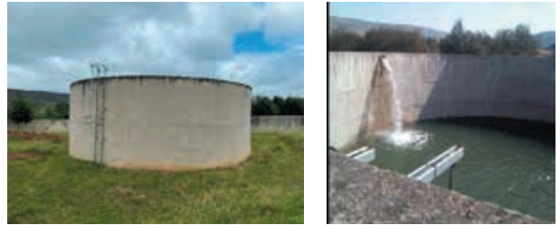
Existing Raw Water Reservoir and Commissioning of such. Water proofing required by specialist sub Contractor.
