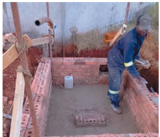
Ulwakhiwo oludala lweMahehle command reservoir inlet chamber. Kuzakufakelwa uphahla lwe-slab, izixhobo kunye nemizila yemibhobho.
