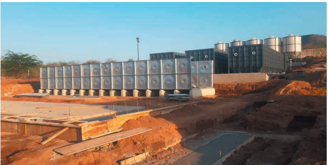
Izicacisi, i-Cougluation kunye ne-flocculation tank, i-Backwashers, itanki yokugcina amanzi acocekileyo, ukulungiswa kweqonga lokucoca isanti kunye negumbi lokwakha iklorine.
