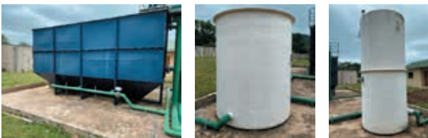
Indawo yokuhlukanisa amanzi: Clarifier, Settled Water Tank, kunye neFlocculation Tank – ziyasebenza.
