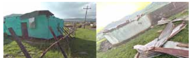
Figure 1 & 2: Depicts Lightning incident and strong wind damage occurred at Dr Nkosazana Dlamini-Zuma LM
